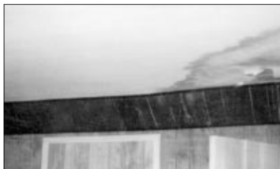
Water damaged this ceiling.
